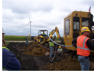
Underground Collector Line
